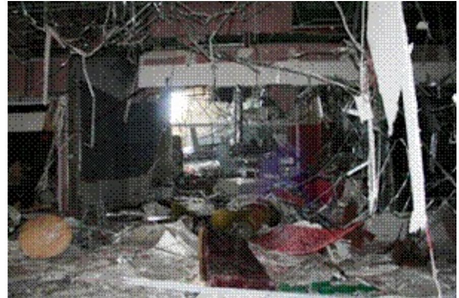
Damages caused by the explosion
