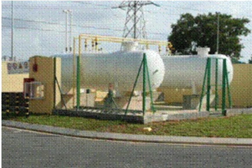
Gas Supply From 2 LPG Tanks
